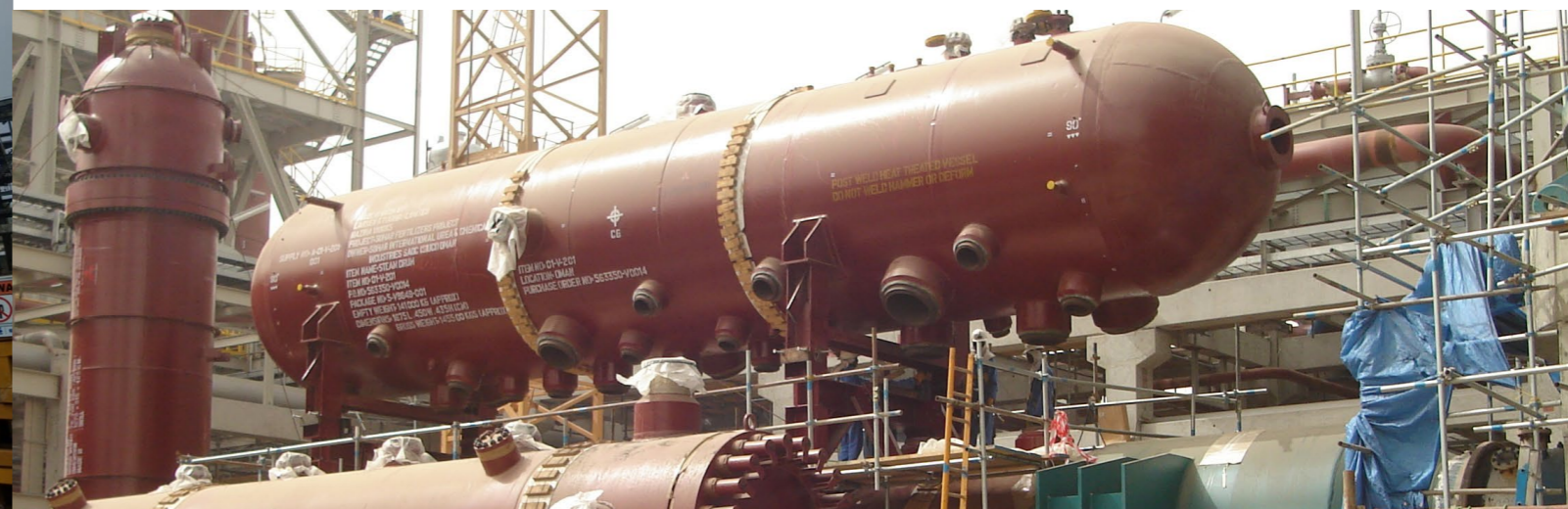
Waste Heat Boiler Package including RG/CG boiler, steam drum, risers & downcomers at Sohar Fertilizer plant
