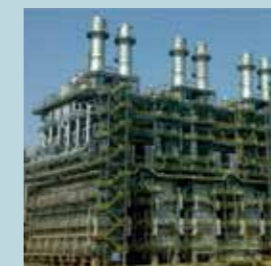
Modular Reformers, Cracking Furnaces & Heaters
