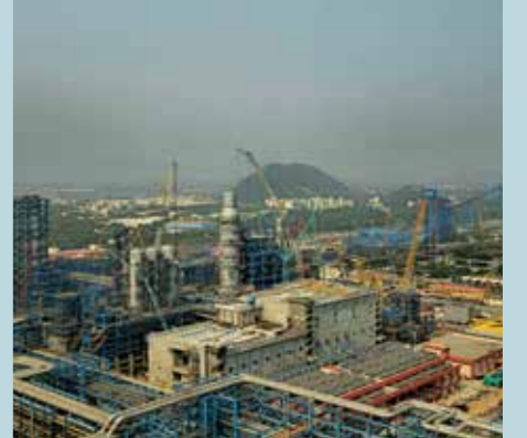
Residue Up-gradation Facility (RUF) Capacity: 3.55 MMTPA | Lummus
