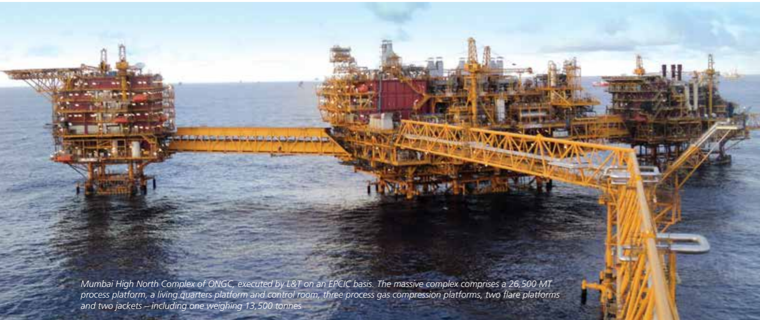
New Water Injection South (NWIS - R) Project for ONGC with 1 st of its kind low saline water injection facility
