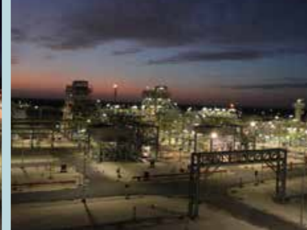
Hassi Tidjerane Field (HTJ) Capacity: 4 MMSCMD
