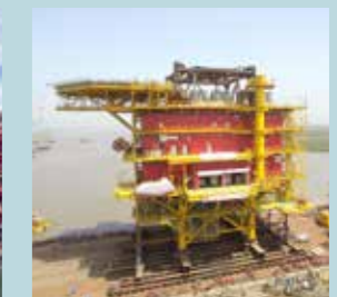
Living Quarter Modules & E-Houses
