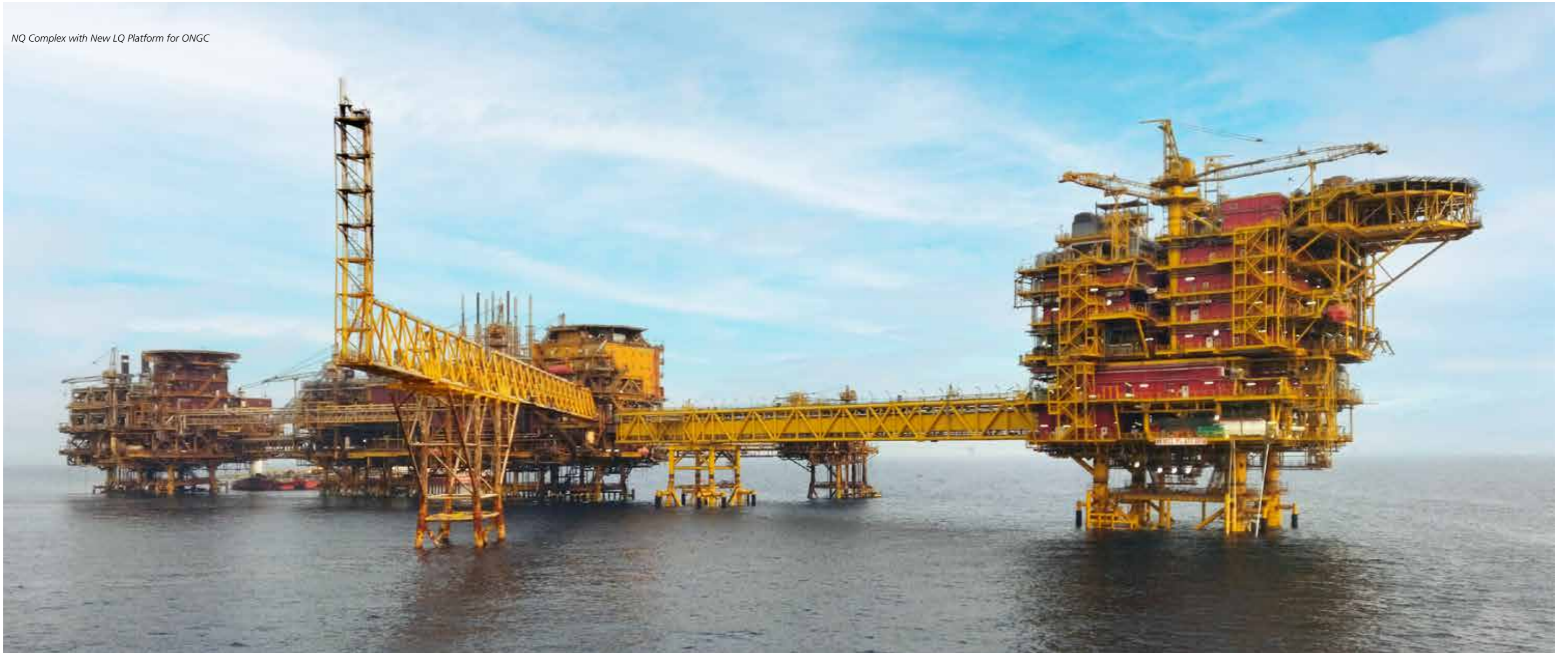
Marine services cover the entire spectrum of offshore installations - LTS 3000 (left), a heavy-lift-cum-pipelay vessel and LTB 300 (right), a pipelay-cum-work barge
