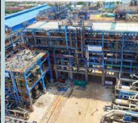
Full Conversion Hydrocracker Unit (FCHCU) Capacity: 3.053 MMTPA | UOP
