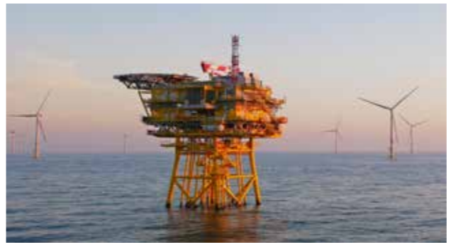
Offshore Substation Platform
