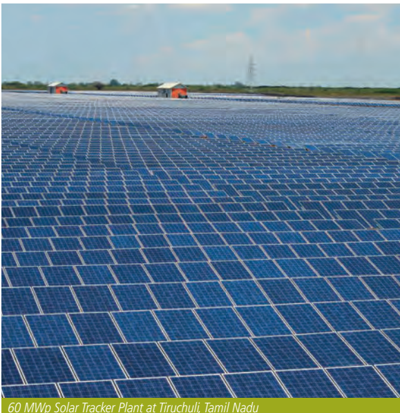
60 MWp Solar Tracker Plant at Tiruchuli, Tamil Nadu
